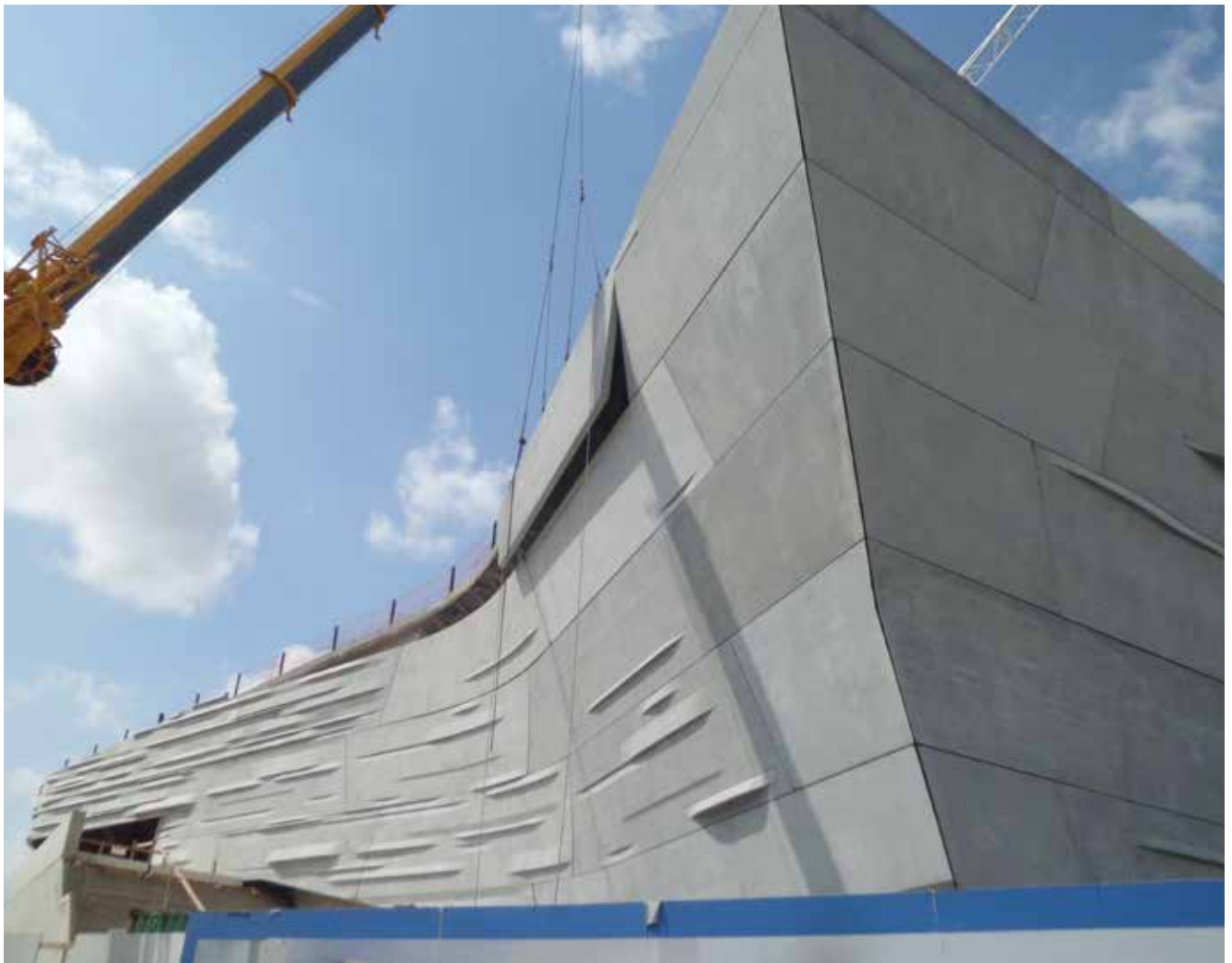
The panels were erected in a careful sequence to avoid overloading one side of the structure. Work began at the base and went around the perimeter, connecting each panel to the next and to the frame. Photo: Gate Precast Co.
